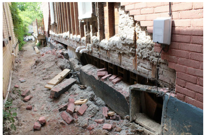
Basement renovation project resulted in partial foundation collapse (Photo credit A. Lohonyai)
